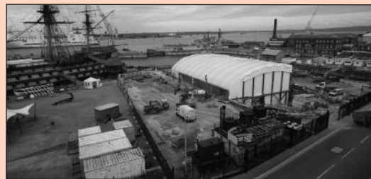
Time-lapse camera footage showing images of the start and completion of the demolition.
